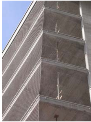
Similar impression created by safety networks of Jakob Rope Systems at a parking garage in Zurich.
